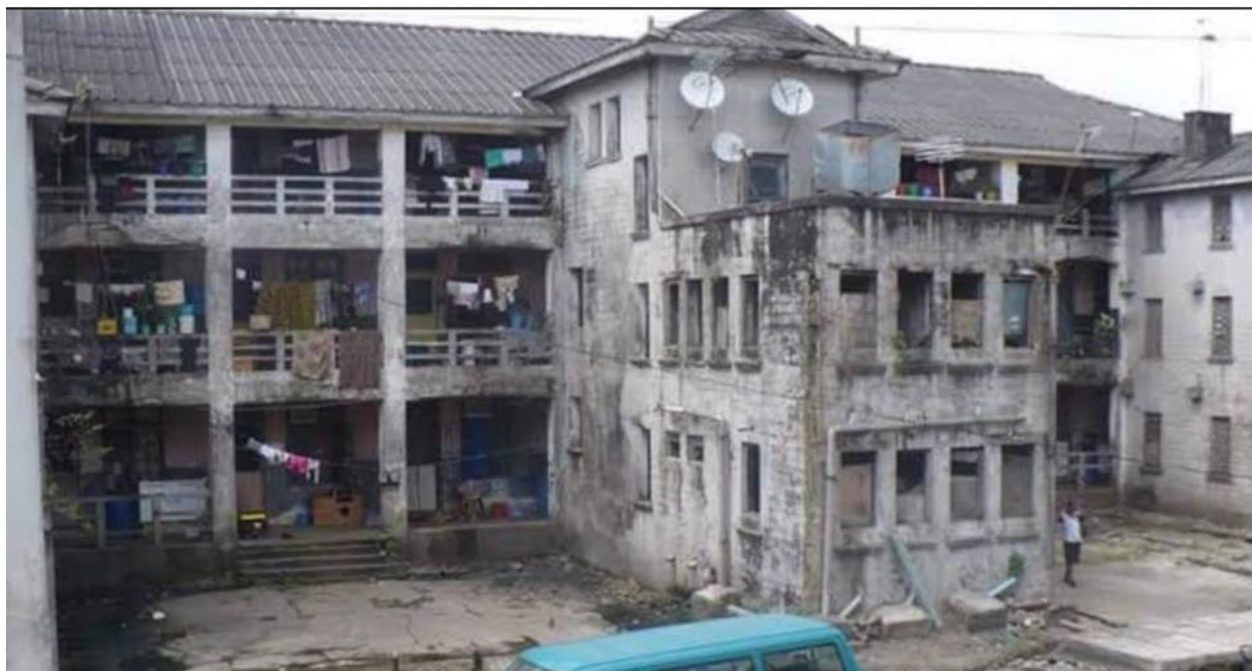
Figure 3: A dilapidated Police Barack in Nigeria
